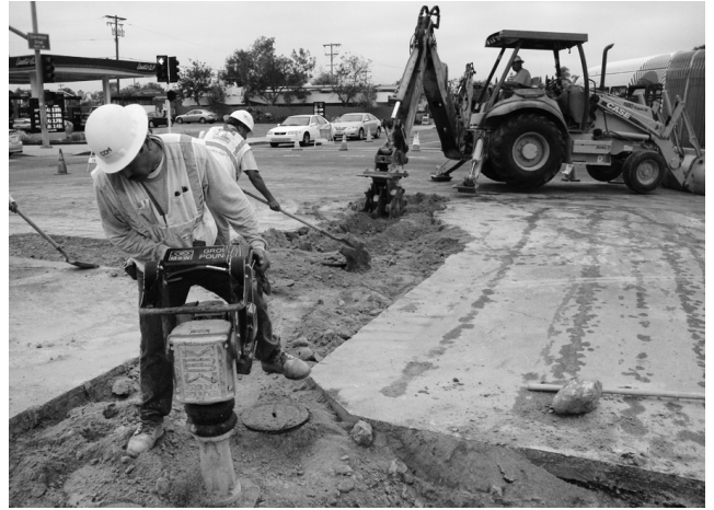
The project 554 team maintained traffic control during construction as shown here at Clairemont Mesa Boulevard and Clairemont Drive.
